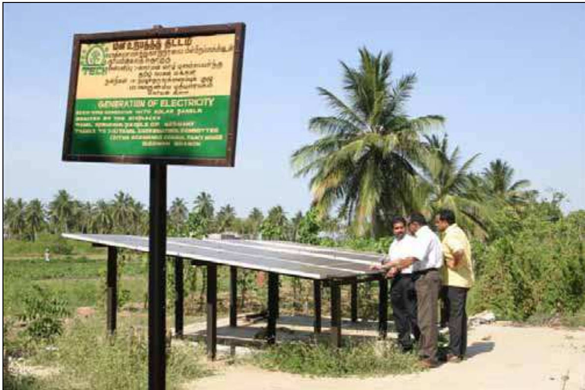
Fig. 2. Solar panel installed in NE-SL
