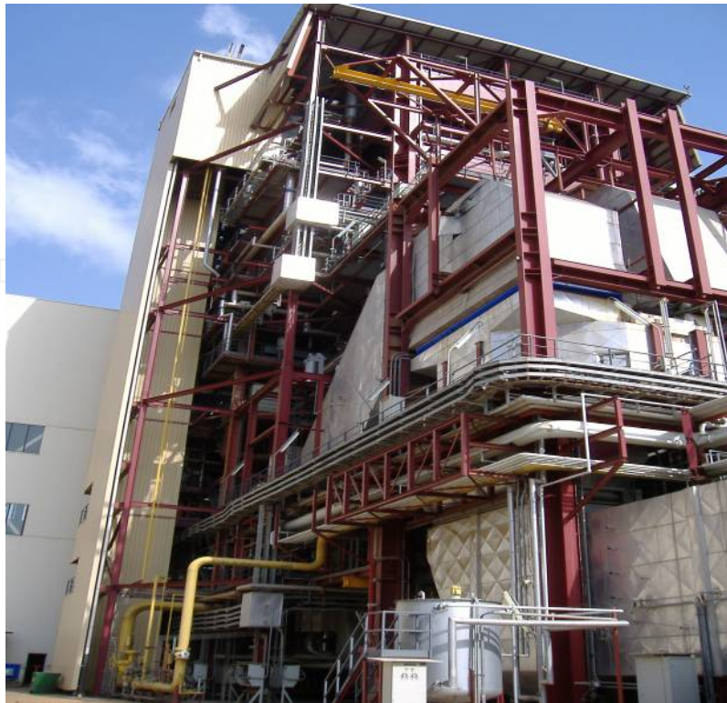
Figure 3. Example of a boiler of a TPP.
