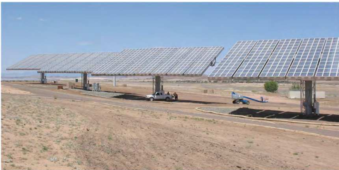
Fig. 2. Several 35-kW CPV systems built by Amonix in Torrance, California were installed at a Public Service power plant in Arizona. The system uses Fresnel lenses to concentrate sunlight onto high efficiency silicon solar cells. The pickup truck in the shade gives an idea of size of this installation.
