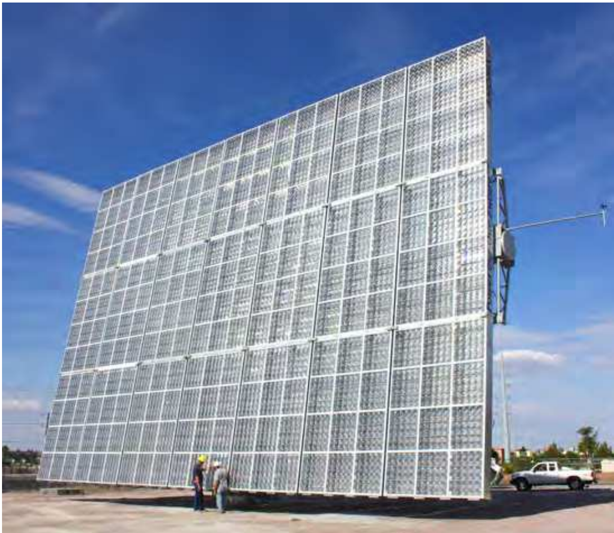
Fig. 4. The Amonix 7700 60 kWac System uses high efficiency multijunction solar cells.
