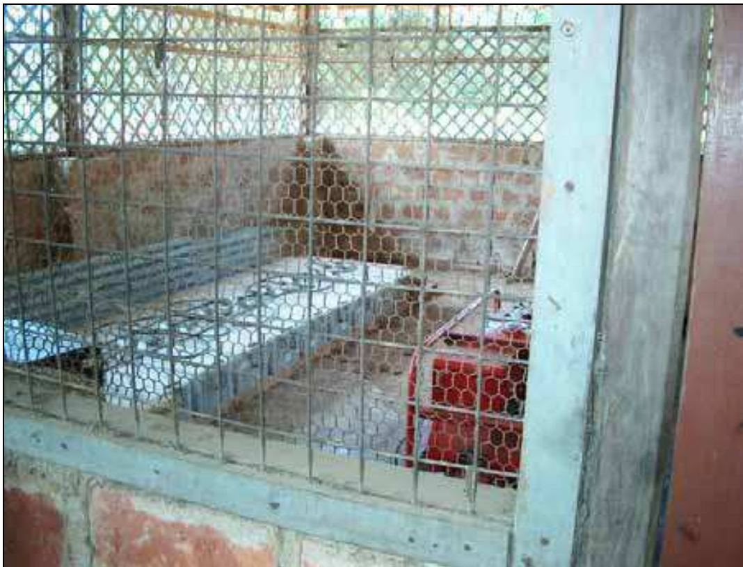
Fig. 4. Battery Storage System
