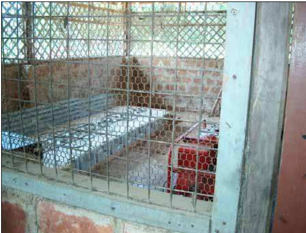
Fig. 4. Battery Storage System
