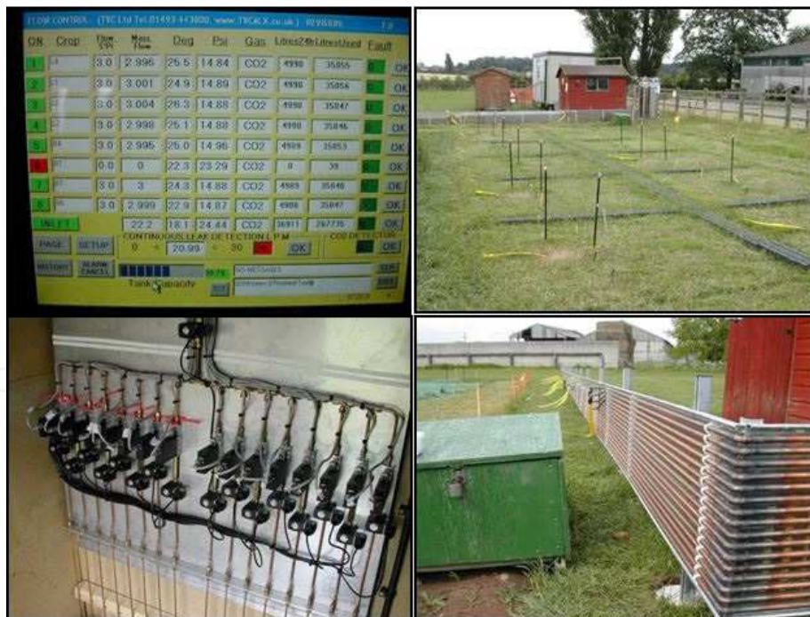
Photo 2. \text{CO}_2 gas delivery hardware and software system installed at the ASGAR site. Top left: automated system to control delivery of gas at a targeted rate, bottom left: copper tubes with automatically controlled valves to supply gas, bottom right: copper tubes are connected to yellow plastic pipes which, in turn, carry gas to individual plots and top right: pasture plots at the ASGAR site with measuring tubes and gas delivery pipes in each plots, and in the back ground the cryogenic gas cylinders and port-cabin can be seen.
