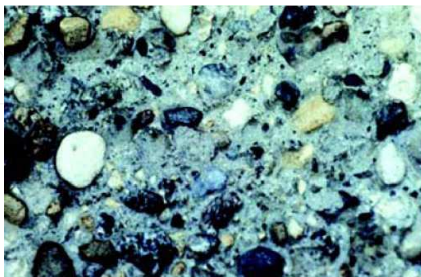
Fig. 1.2. Concrete disintegration due to abrasion [7]
