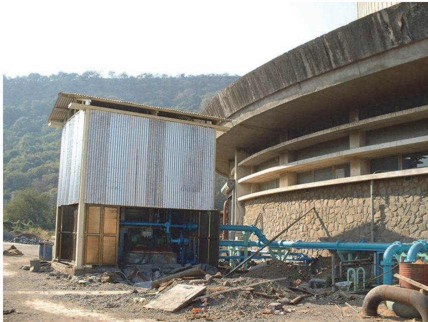
Fig. 4. Desalination unit located outside Cirus annulus area
