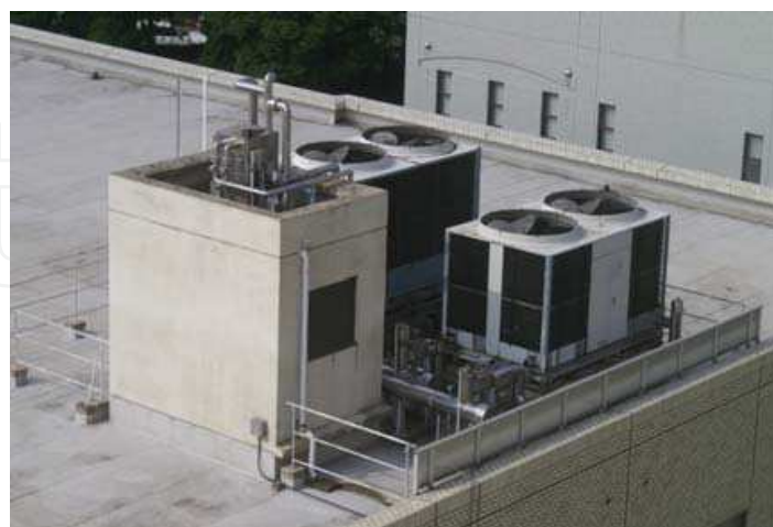
Fig. 14. Heat pump - chiller units
