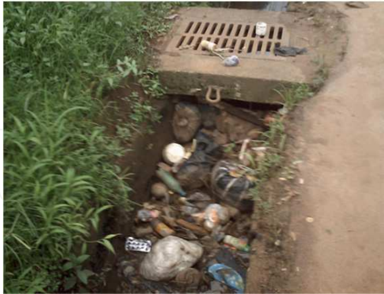
Fig. 7. Solid waste accumulated in the entrance of a manhole of a drainage system
